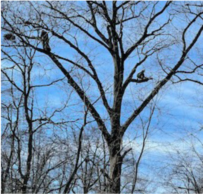
DTE tree trimmers work high above the electric power lines clearing limbs.
